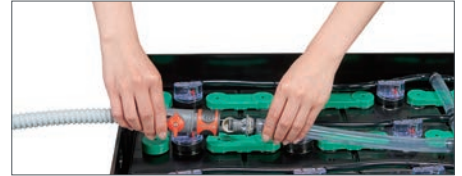
Refilling preparation: Snap-connect the couplings of the hoses on the tank and battery sides and open the faucet.
