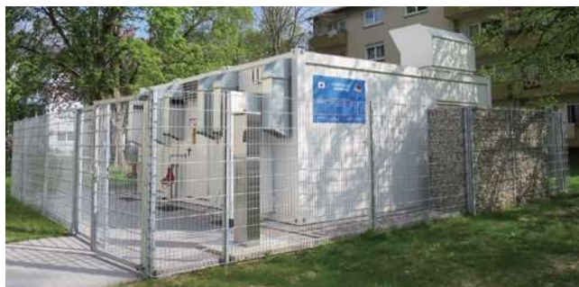
図2 実証システム外観 Figure 2 External view of the demonstration system
